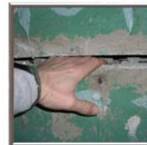
Major Wall Crack
