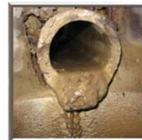
Muddy Drain Tile
